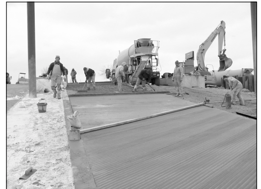
No. 8 coarse aggregate in concrete mix facilitated sharp definition of ODNR's v-grooved surface for new boat ramp in Buck Creek State Park.
